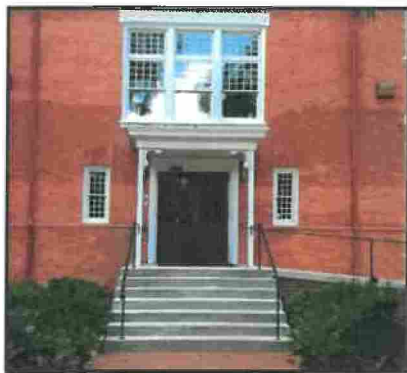
These stairs will be removed and replaced.
