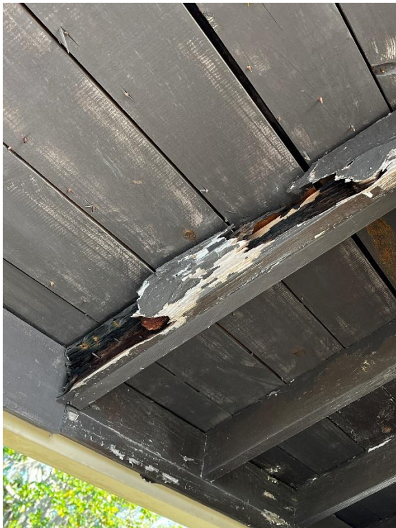
Rotten wood at eaves
