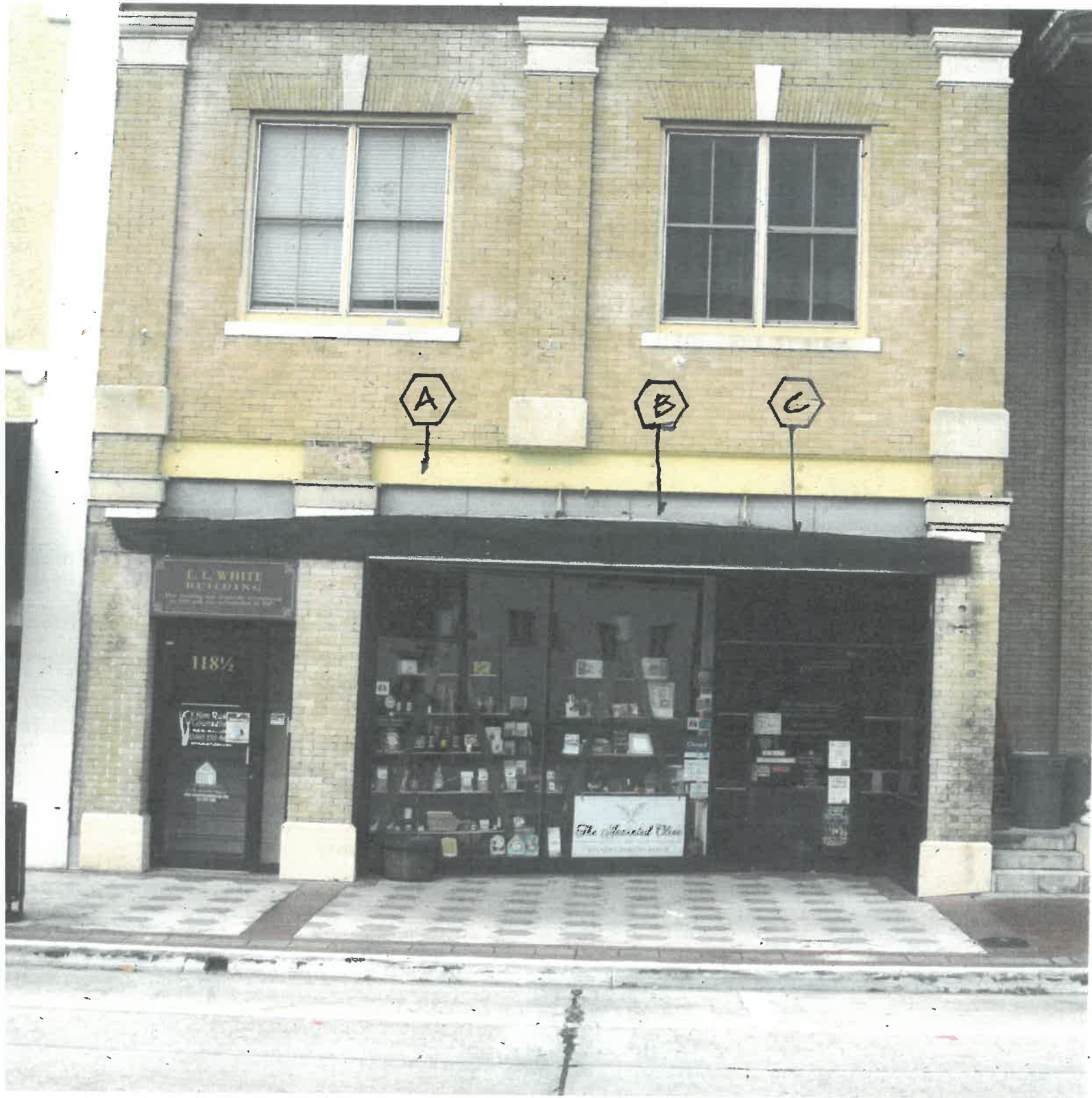
EXISTING FASCIADE CONDITIONS AFTER DEMOLITION OF THE FORMER CANTILEVERED ROOF WHICH PROJECTED OVER SIDEWALK.
