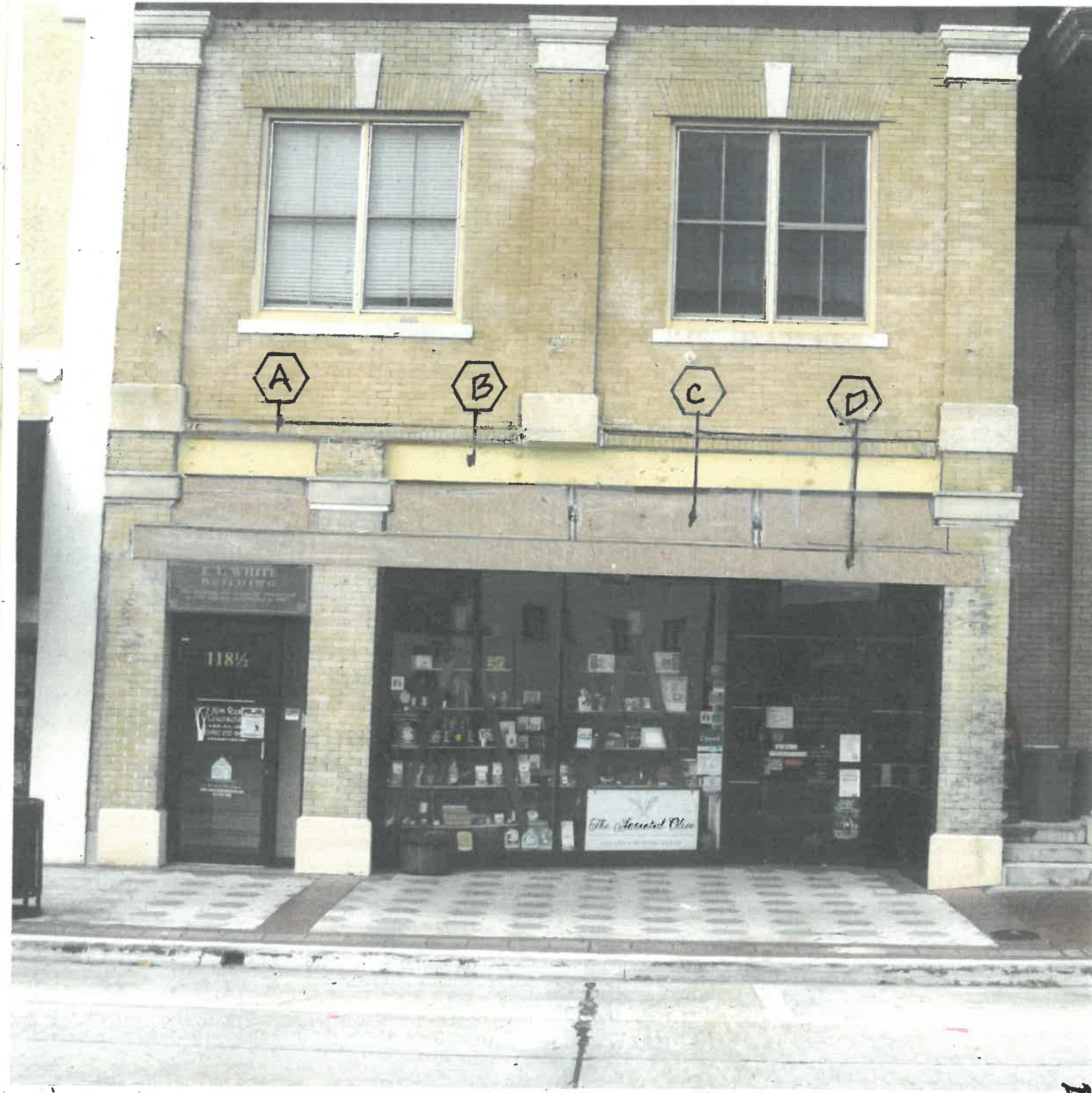
PROPOSED MODIFICATIONS TO EXISTING FASCIADE FOR PURPOSES OF PROVIDING STRUCTURALLY SOUND ELEMENTS NEEDED FOR ATTACHMENT OF PROPOSED AWNING (NOT SHOWN FOR CLAIRITY). PROPOSED AWNING WILL VISUALLY BLOCK TRANSOM ELEMENTS FROM VIEW.
