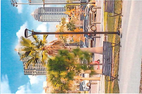
PEDESTRIAN LIGHTING - MILLLENIA
