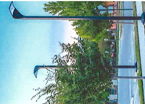
SITE LIGHTING - MILLENIA FIXTURE
