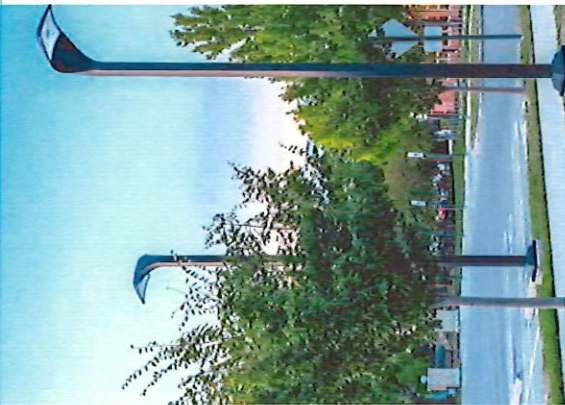
SITE LIGHTING - MILLENIA FIXTURE
