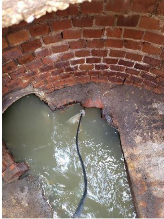
Figure 4.3 Back Flow from the 15" incoming pipe at Site 3
